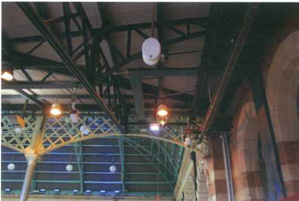
Figure 2: Detail view of truss structure of platform access area roof adjacent to the East Wing of the Main Terminus.
